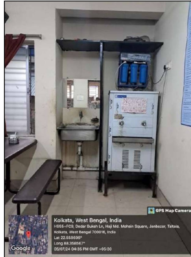
DRINKING WATER-CUM-COOLER FACILITIES
