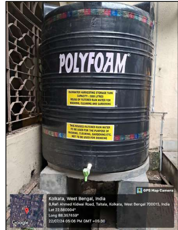
RAINWATER HARVESTING UNIT FOR RAINWATER STORAGE AND REUSE
