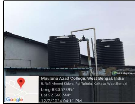
OVERHEAD WATER TANKS IN COLLEGE ROOFTOP
