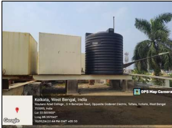
OVERHEAD WATER TANKS IN COLLEGE ROOFTOP
