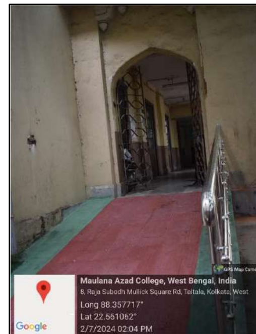
RAMP 2 WITH TACTILE PATH AND RAIL LEADING TO COLLEGE HALL AT GROUND FLOOR
